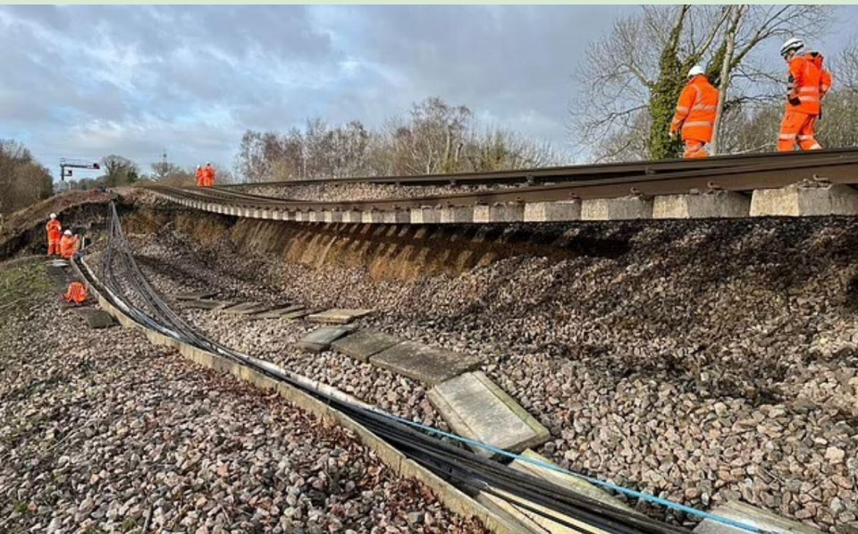
Hook Line collapse (Wok-Bas)
